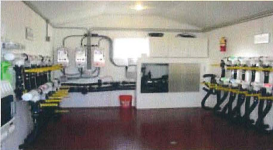
“McHenry County Blending Facility”
