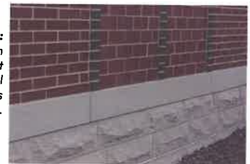
Figure C5.3.ivb: Brick veneer is in laid in pre-cast panels. Vertical articulation features mask the joint lines.
