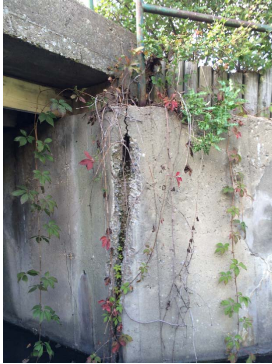
Photo No. 7 – Crack in Wingwall Joint
