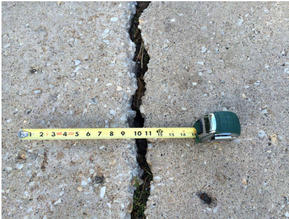
Photo No. 4 – Largest Crack is full depth
