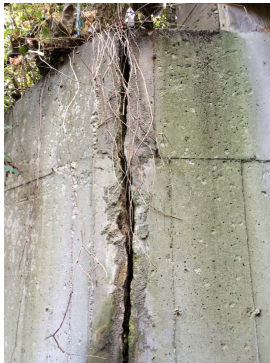
Photo No. 8 – Cracks in Wingwall Joint
