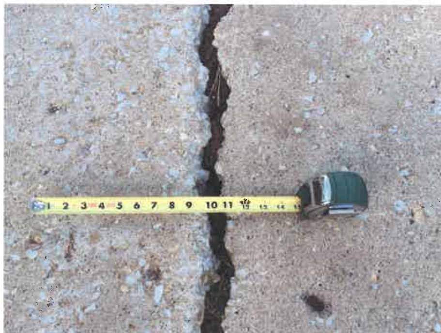
Photo No. 4 – Largest Crack is full depth
