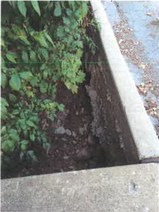
Photo No. 5 – Roadway undermining northwest corner
