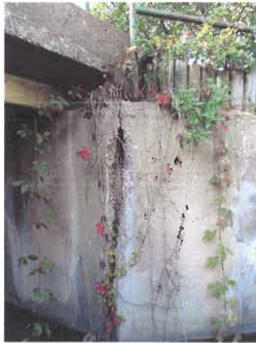
Photo No. 7 – Crack in Wingwall Joint
