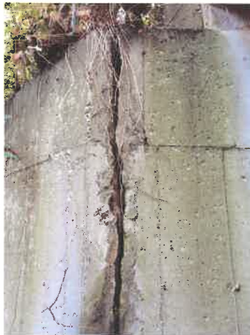
Photo No. 8 – Cracks in Wingwall Joint
