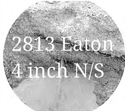
Leak on 4" CI Main Line
