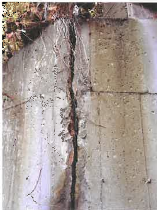
Photo No. 8 – Cracks in Wingwall Joint
