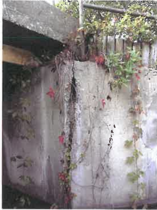
Photo No. 7 – Crack in Wingwall Joint
