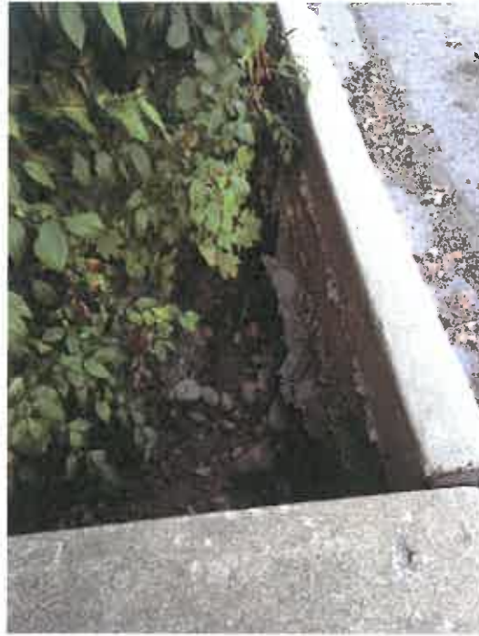
Photo No. 5 – Roadway underming northwest corner
