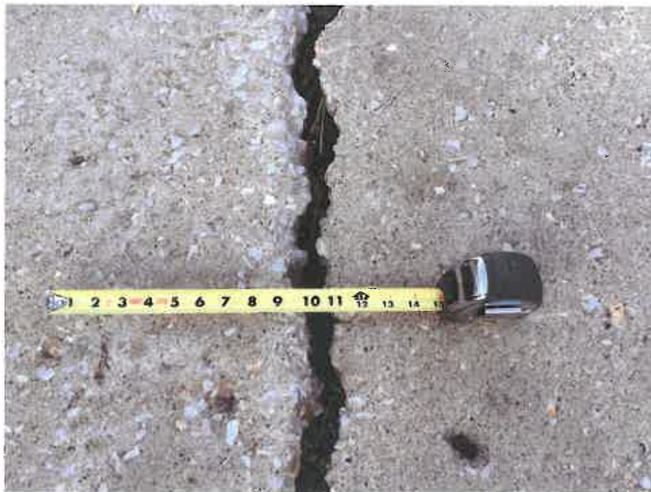
Photo No. 4 – Largest Crack is full depth
