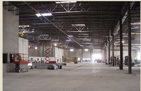
Work progresses on the fleet maintenance area of the new Public Works Service Center.
