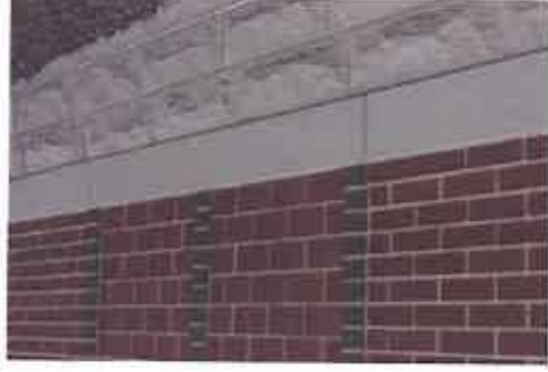
Figure CS.3.ivb: Brick veneer is laid in pre-cast panels. Vertical articulation features mask the joint lines.
