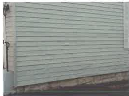
Fig. 36: Vinyl and aluminum siding are discouraged materials and should not be used to cover historic building materials
