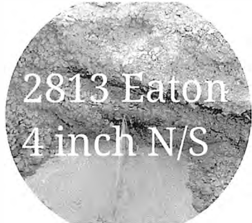
Leak on 4" CI Main Line
