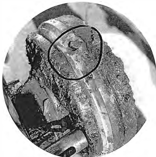
Leak on Corroded Hydrant Shoe
