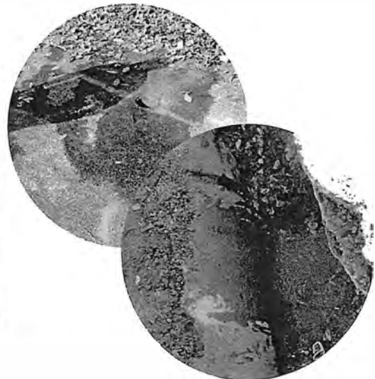
Leak on AC Main Line
