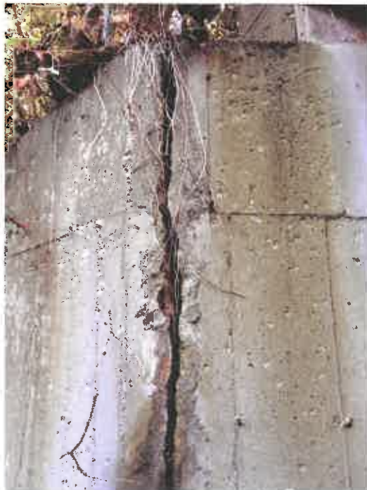
Photo No. 8 – Cracks in Wingwall Joint
