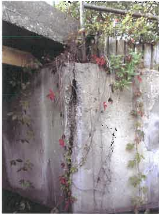
Photo No. 7 – Crack in Wingwall Joint
