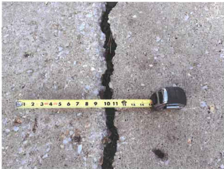
Photo No. 4 – Largest Crack is full depth
