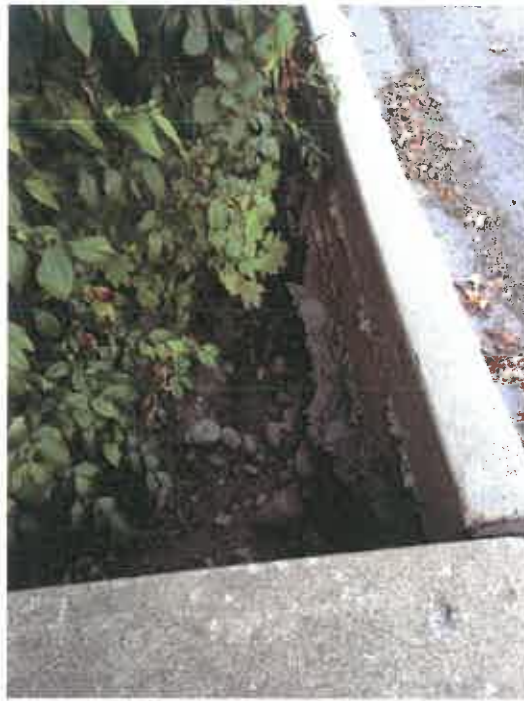
Photo No. 5 – Roadway undermining northwest corner
