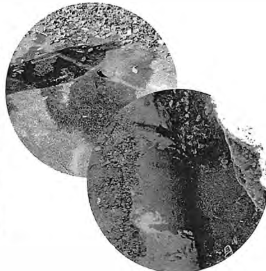
Leak on AC Main Line
