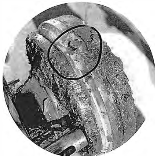
Leak on Corroded Hydrant Shoe
