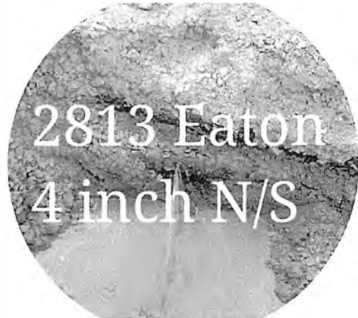
Leak on 4" CI Main Line
